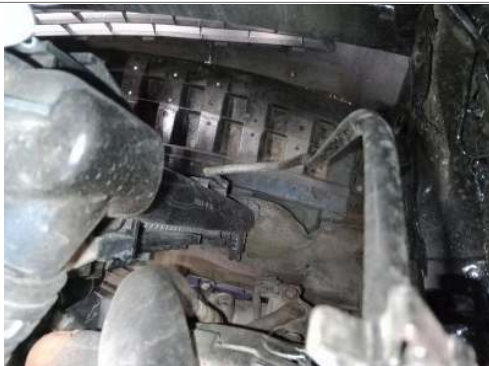
Air conditioner pipes
