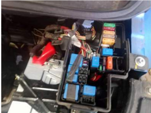
Fuse box cover missing
