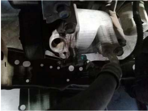
Air conditioner pump
