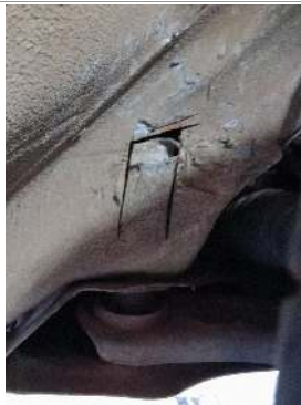
Main Beam Right
