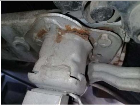
Main Beam Right
