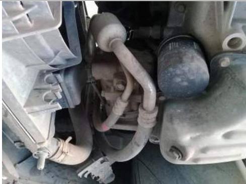
Air conditioner pipes
