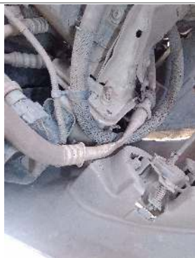
Air conditioner pipes
