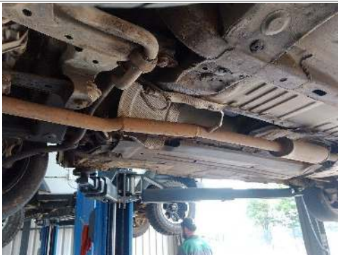
Engine to silencer pipe
